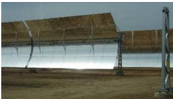
Andasol 2 x 50 MW, Guadix
