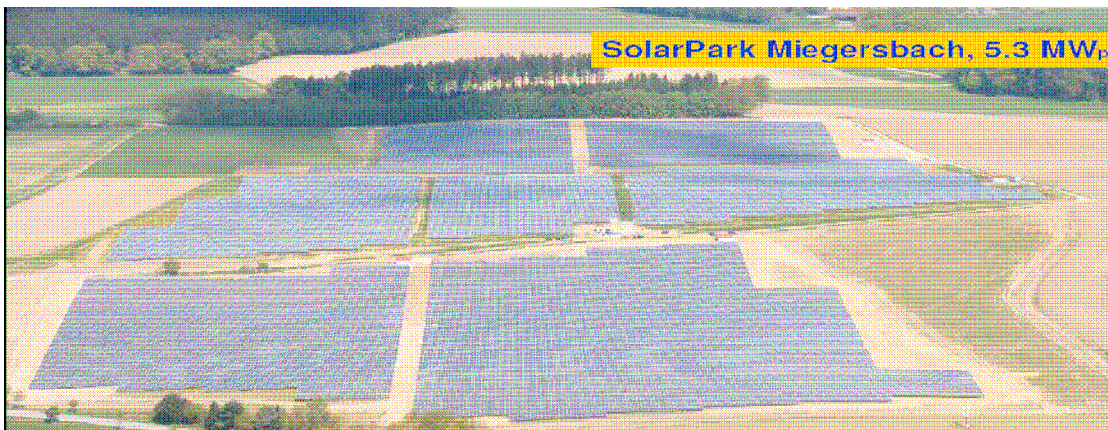
PV-power generation plant
